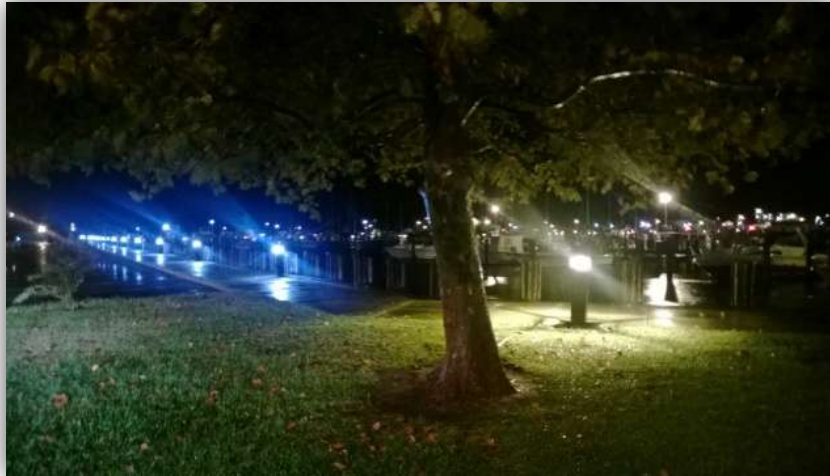
New energy efficient lighting in place at Somers Cove.
