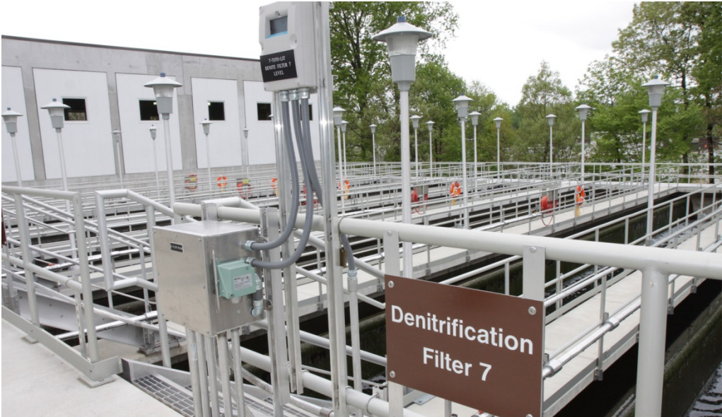
The Enhanced Nutrient Removal Expansion and Improvements project at the Little Patuxent Water Reclamation Plant reduces the amount of nutrients released to the Bay.
