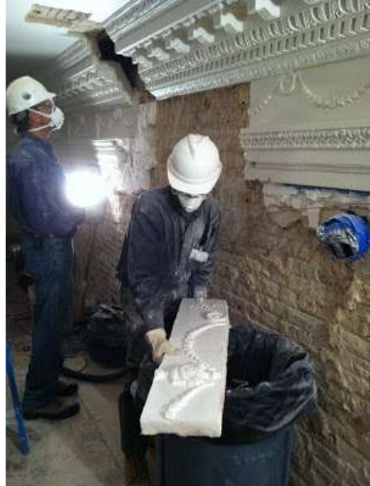
(Preservation specialists from the firm of J.M. Kelley, Ltd., remove sections of the 1905 entablature to reveal evidence of the original form and height of the cornice and ceiling. Once removed, these elements are being catalogued and stored by the DGS.)
