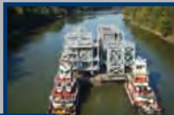
Left: The modular units for the CO2 capture facility were assembled in Tuscaloosa, AL, and barged down the Mobile River for delivery at Plant Barry in Bucks, AL.
