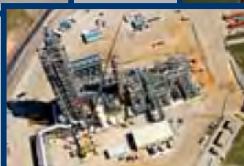
Right: Construction of CO2 Capture unit at Alabama Power's Plant Barry in Bucks, AL.
