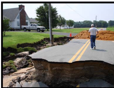
An entire section of Indiantown Road washed away in Dorchester County as a result of flooding in 2006.
