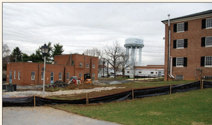
Preliminary ground work begins before the demolition of the old Heating Plant, left, and Barry Hall, right.
