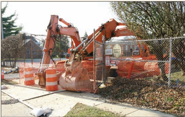
Heavy equipment used to unearth water line blocks entrance to Bjorlee Parking Lot.
