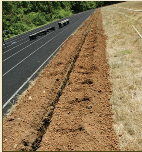
Old field was sprayed to kill all growth and irrigation system is installed.
