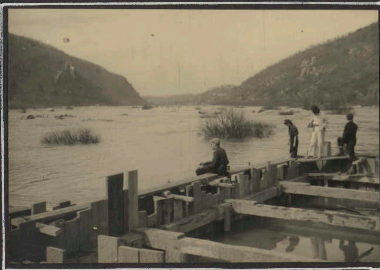
IN THE MIDDLE OF THE POTOMAC OFF SANDY HOOK. "CONSTRUCTION" FOR PIERS OF NEW BRIDGE
