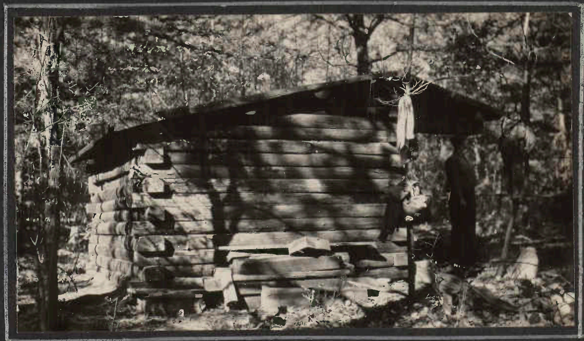
AND SO THE SHELTER SHAPED UP THUS AT THE END OF THE DAY --
