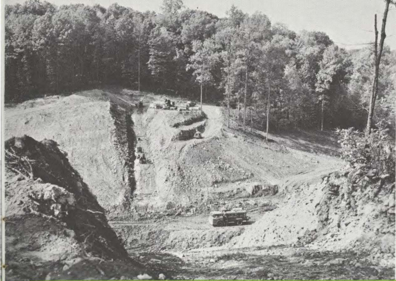
Construction continued through the fall and winter, with the bowl at the dam site dwarfing the men and equipment of Harris & Brooks, Inc., Laurel, Md., winners of the construction contract. Height from base to top of the earth dam was to be 55 feet when it was completed.
