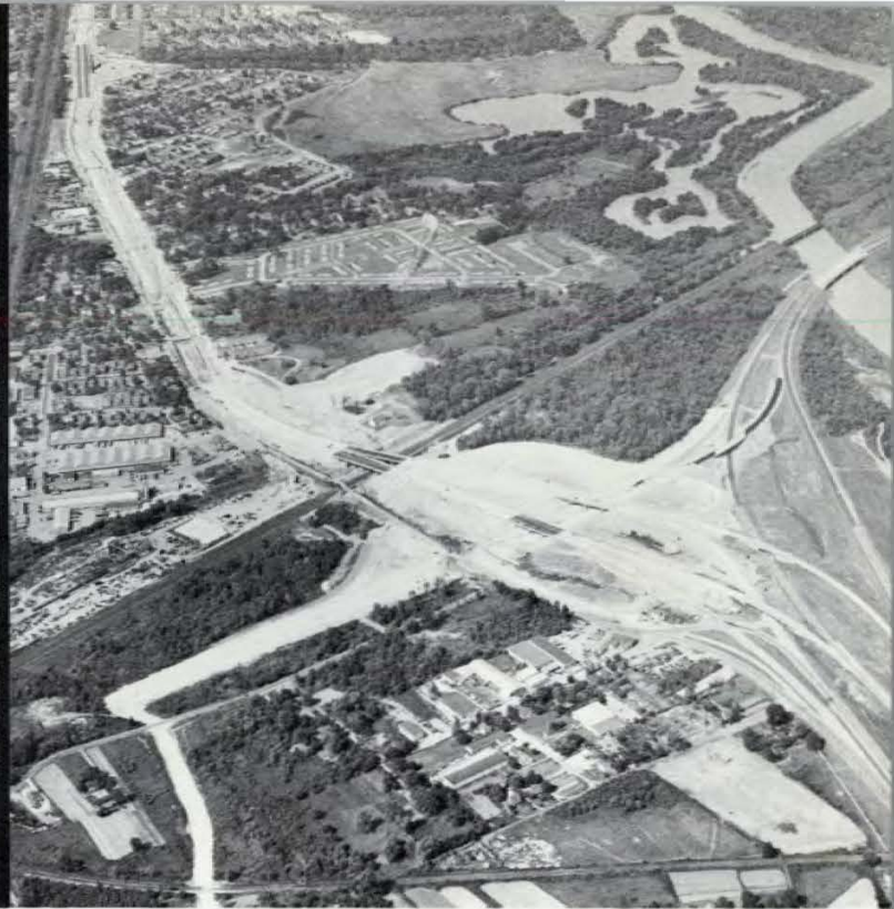
The nearly completed Kenilworth interchange, the intersection of three major highways — Kenilworth Avenue, the Annapolis Expressway, and the Baltimore-Washington Parkway.
