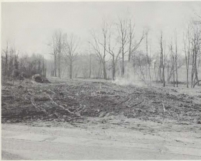
Clearing land for the parkway extension —looking south from Old Bladensburg Road.
