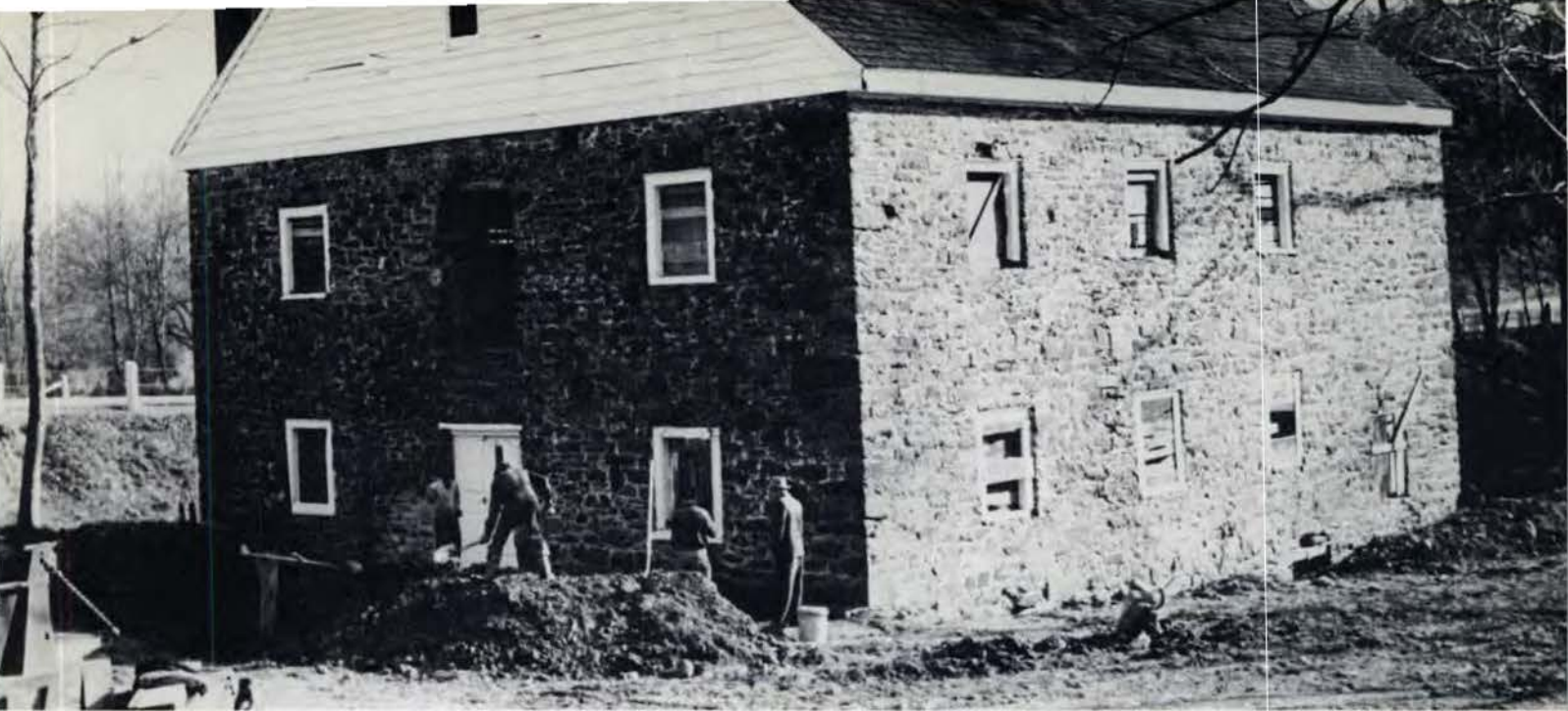
Commission workmen digging ditch around the 150-year-old Adelphi Mill in Northwest Branch Park preparatory to waterproofing and repairing the historic structure. The Commission plans to make at least a portion of the mill available for community and recreation use. The building is on Riggs Road about three-quarters of a mile north of University Lane.
