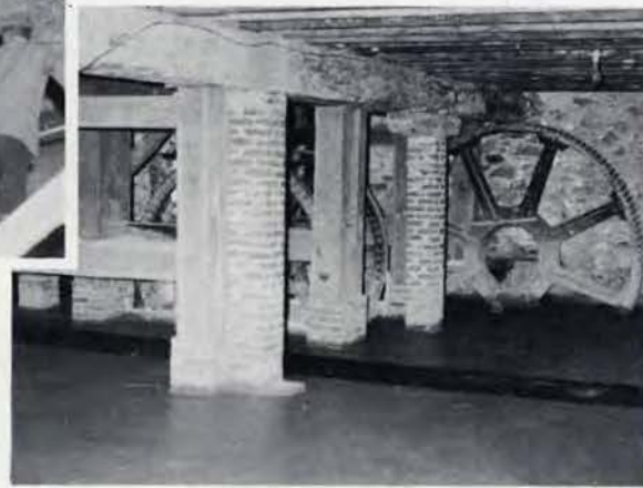
Here is the basement of the mill after it was cleaned and a concrete floor installed.
