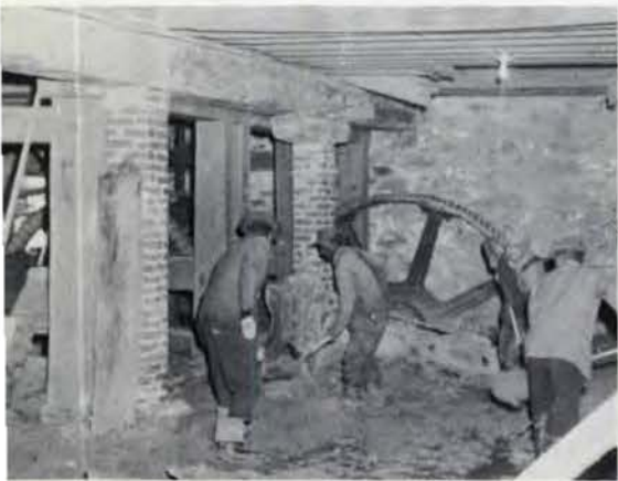
This is how the basement of the mill looked in December, 1953, when the Commission workers began cleanup operations.
