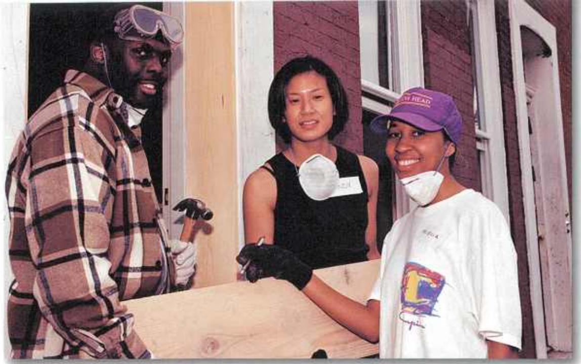
James Thomas, Cindy Hung and Felecia Baker work as a team on an interior construction project at a house on Fulton Avenue in Baltimore City.
