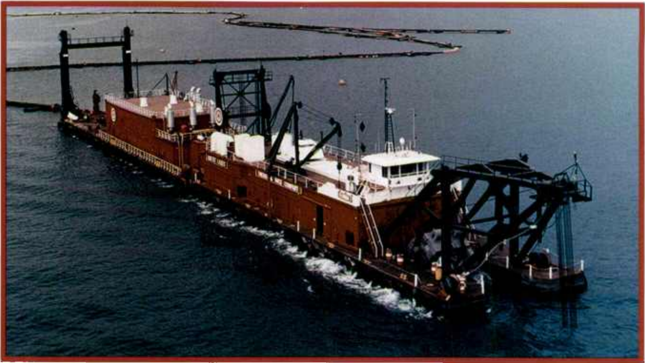
The Florida at work on the Pier J Expansion project in the Port of Long Beach, California.
