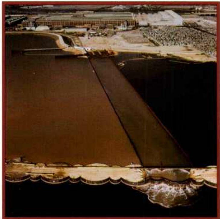
Strict turbidity standards required the construction of several treatment ponds and a special settling basin, where flocculants were employed to assure cleansing of the effluent before its return to the river.
