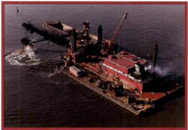
In New York/New Jersey Harbor: The Chicago was the primary dredging tool used in the deepening of New York New Jersey Harbor, the largest dredging contract in the history of the U.S. Army Corps of Engineers.
