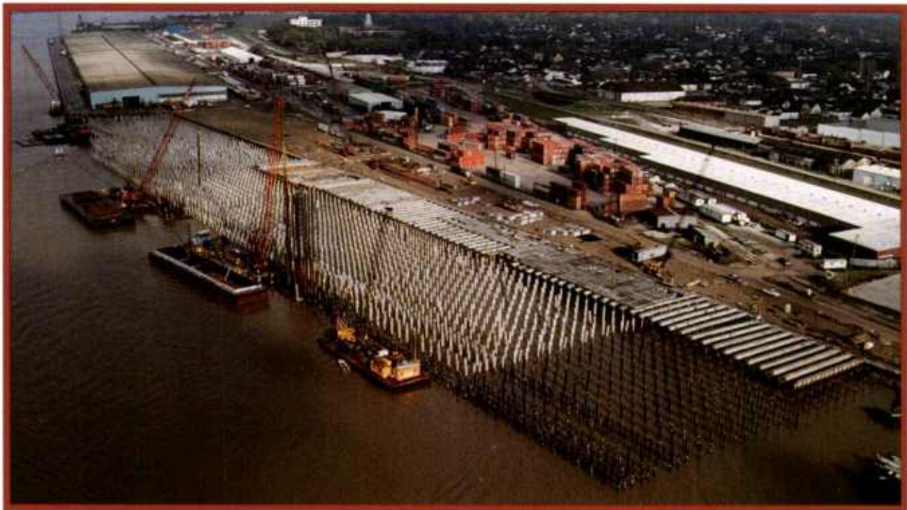
A total of 4,640 tubular steel and steel-reinforced concrete piles were required for Nashville Ave. Wharf.
