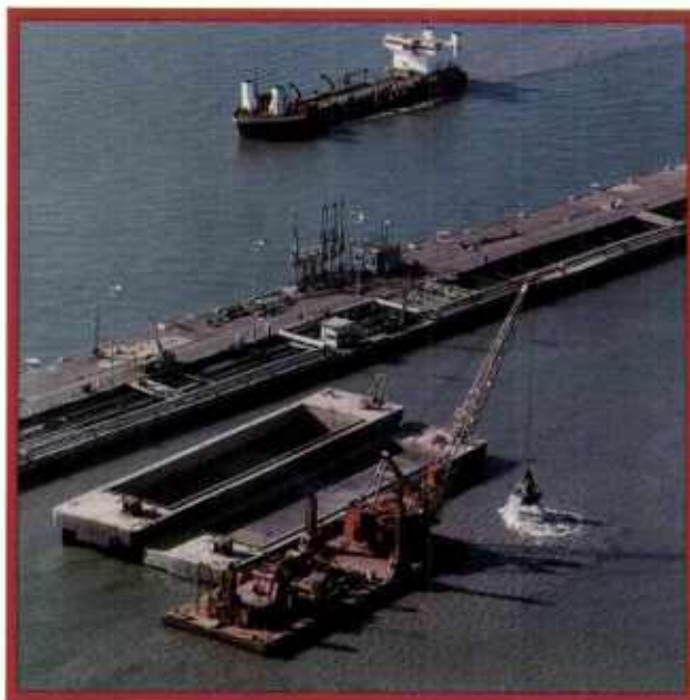
Joint work: Dredge No. 53 is shown in San Francisco Harbor performing maintenance work. The company's trailing suction hopper dredge Padre Island is dredging material on the dock's outer side.
