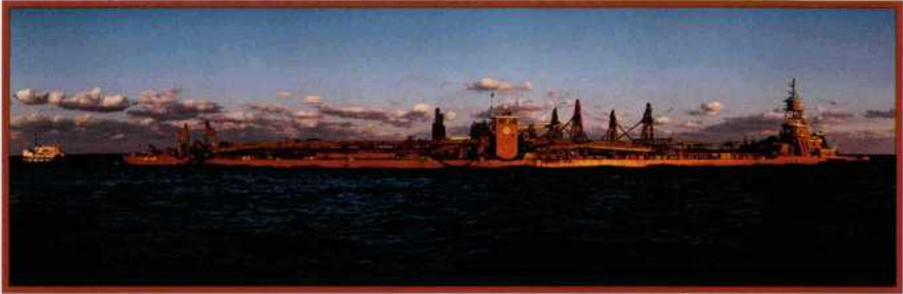
The trailing suction hopper dredge Long Island, a tug-integrated dredge, worked on both phases of the project.
