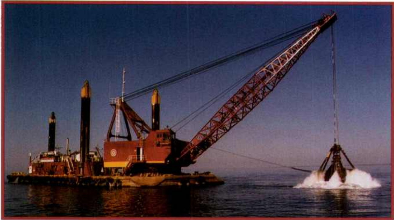
Pipeline crossing: Dredge No. 54 excavates material from the bottom of Long Island Sound for a gas pipeline. The material was sidecast, later to be rehandled in covering the pipeline. Electronic positioning and production monitoring equipment aid in this precise work.
