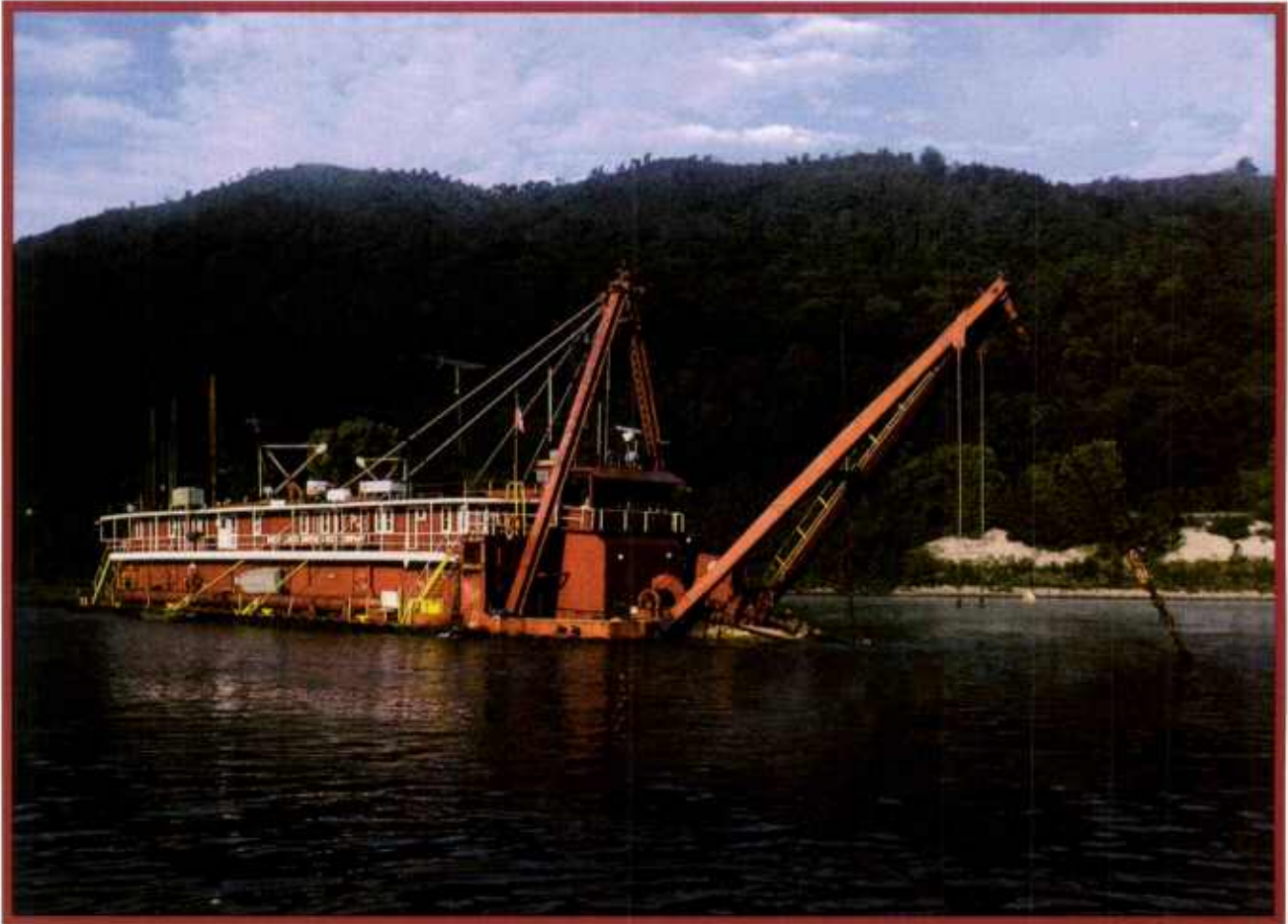
The Louisiana performs maintenance work on the Kanawha River in connection with annual Ohio River maintenance work.
