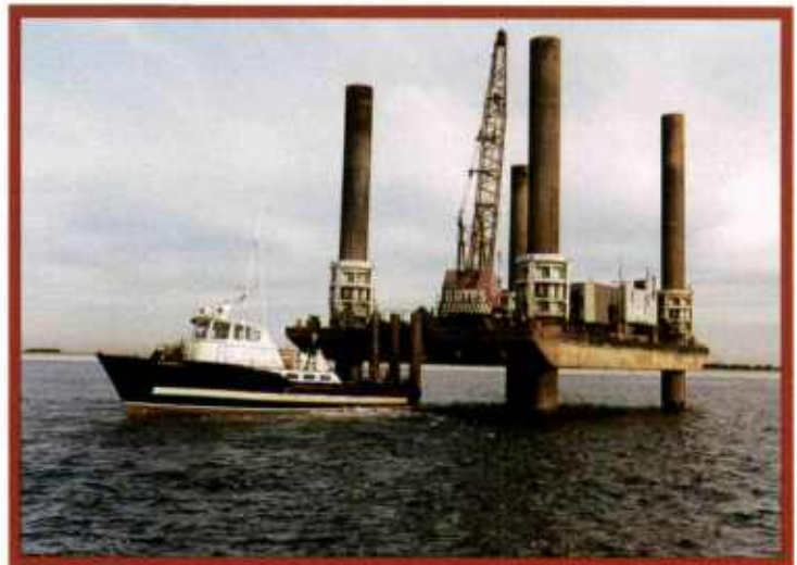
Gates' jack-up barge provides a stable platform for heavy lift and other work.
