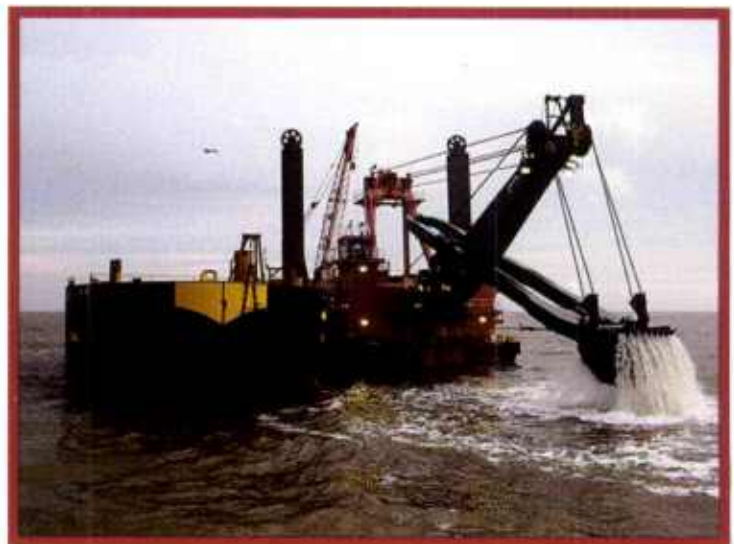
As a dipper dredge, the Chicago can dig in unblasted rock, though she more frequently works in conjunction with Great Lakes' fleet of drill boats, removing rock that has been broken by drilling and blasting.
