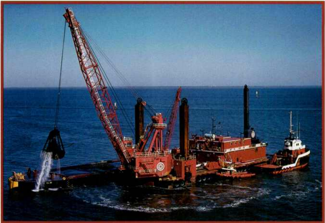
The Chicago offshore at Mobile, Alabama, on her first major project. Great Lakes' leadership in the clamshell (grab) dredging market is a result of the company's commitment to build and maintain the finest, most efficient equipment.
