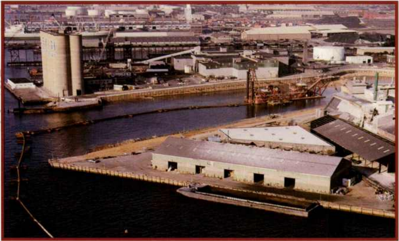
Tunnel Trenching: The dredge Illinois (above) excavates a deep trench into the river bank to provide for the flotation and installation of the steel tunnel tube sections.
