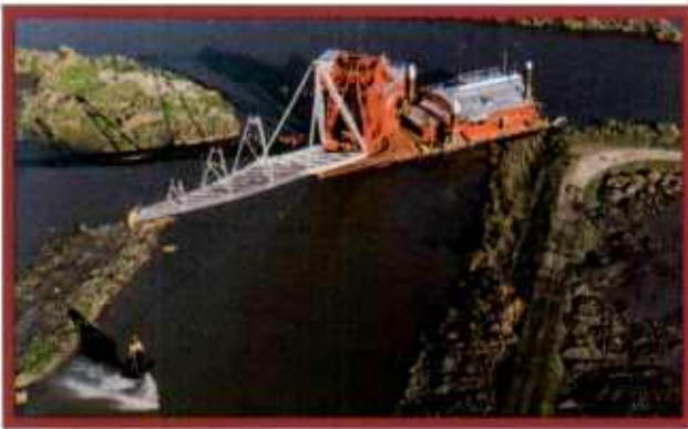
The Conical at work on the storm protection system on the Bayou Lafourche in Louisiana.
