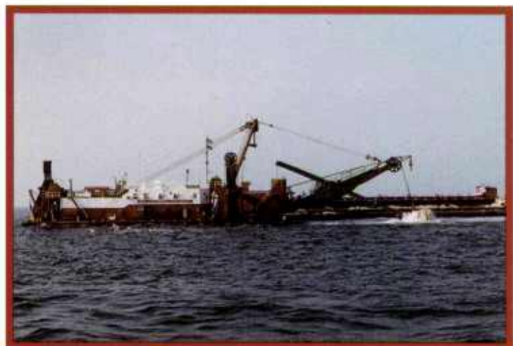
In dipper mode, the Boston works in Dubai on the Jebel Ali project.
