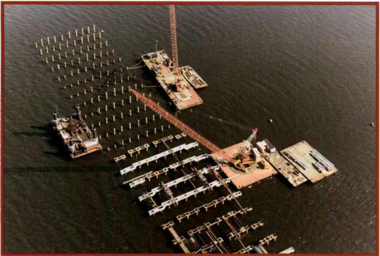
Ringer and derricks position caps atop pilings for the ammunition pier and trestle erected for the U.S. Navy at Colts Neck, New Jersey.
