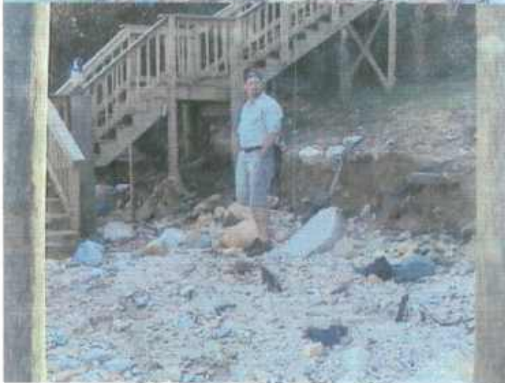
eroded cliff from storm surge 2
