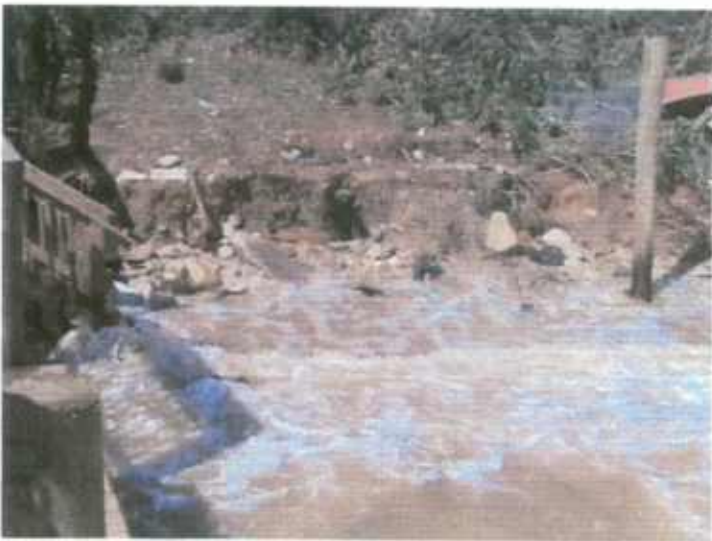
eroded cliff from storm surge 1
