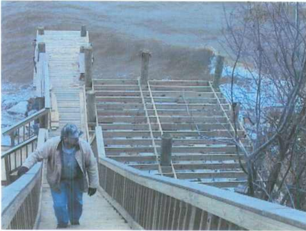
The platform is attached to the pilings that support the stairs, landing and pier and to the pilings for our boat ramp/launch.
