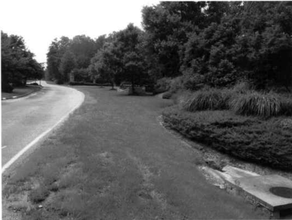
Photograph #2. Looking west down existing utility right-of-way, showing existing storm drain manhole.
