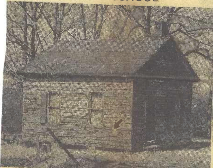
Note loose boards on walls of building.
