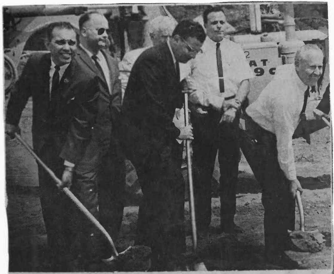
DIGGING IN FOR PRINCE GEORGE'S--Wielding shovels of ground breaking ceremonies for a new State Roads Commission building of Greenbelt are (l-r) State Senator Fred L. Wineland (D., Pr. Geo's.), William C. Birely, of the Montgomery County Council, and State Comptroller Louis Goldstein. The $780,000 building will be erected on a site at the intersection of the Capital Beltway (Interstate 495) and Kenilworth Avenue (Rt. 201).-Photo by Rog White.
