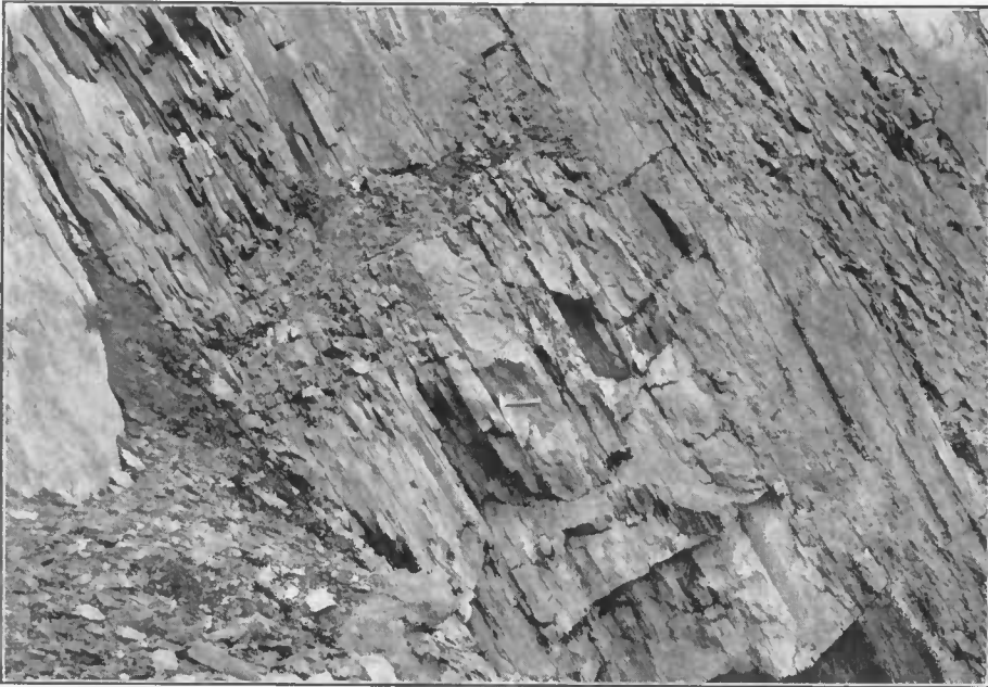
FIG. 2.—VIEW SHOWING THE CONTACT OF THE KEYSER MEMBER OF THE HELDERBERG WITH THE TONOLOWAY LIMESTONE AT KEYSER, W. VA.
