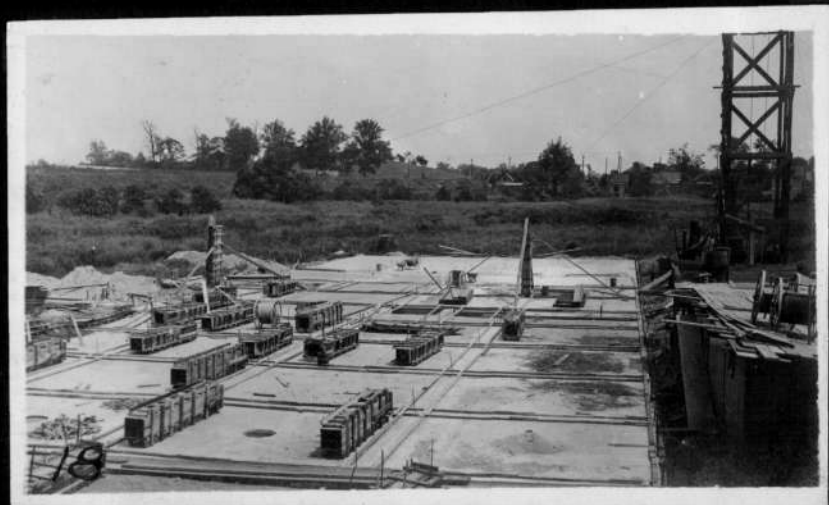
Werk Soap Co. Second section of North Bld., templates laid ready for erection of col.
