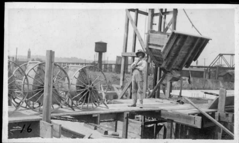
Werk Soap Co. Bridge connecting the two buildings. Used for the concrete buggies.
