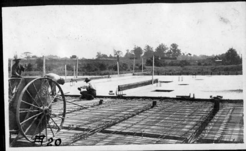
Werk Soap Co. Slab steel. Note stops in beams also note 2x6 planks bolted to col. steel, used in leveling slab.
