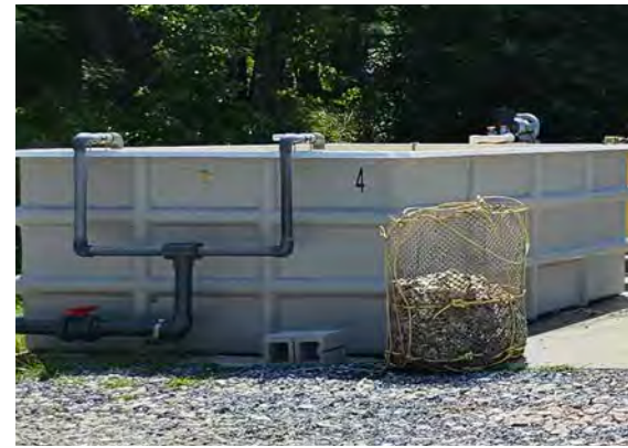
Four fiberglass remote setting tanks purchased by
