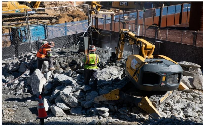
Work crews resumed construction near the Bethesda Shaft, which will provide access to both the Purple Line and WMATA's Red Line.
