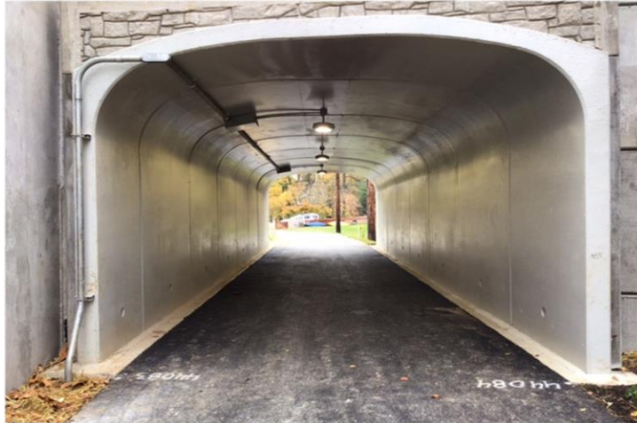
Crews completed the Seaford Road underpass in Chevy Chase, a key access point for local high school students and other pedestrians.
