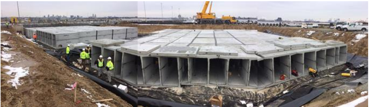
Fairfield Marine Terminal Wet Basin, Underground Storm Water Management System, January 2019.
