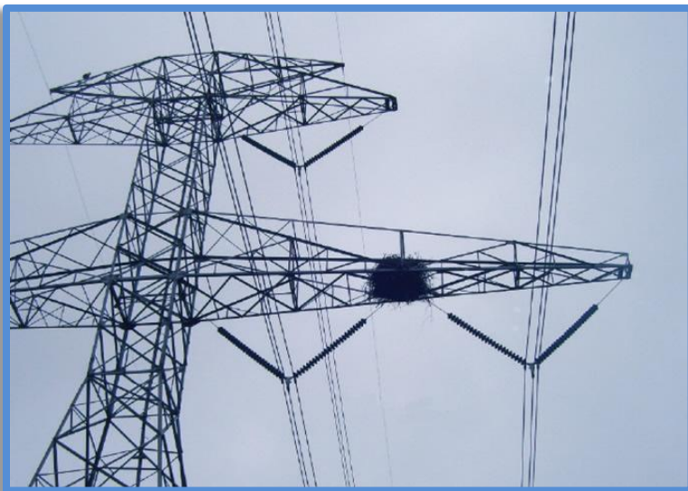
Figure 4-23 Bald Eagle's Nest in a Transmission Tower
