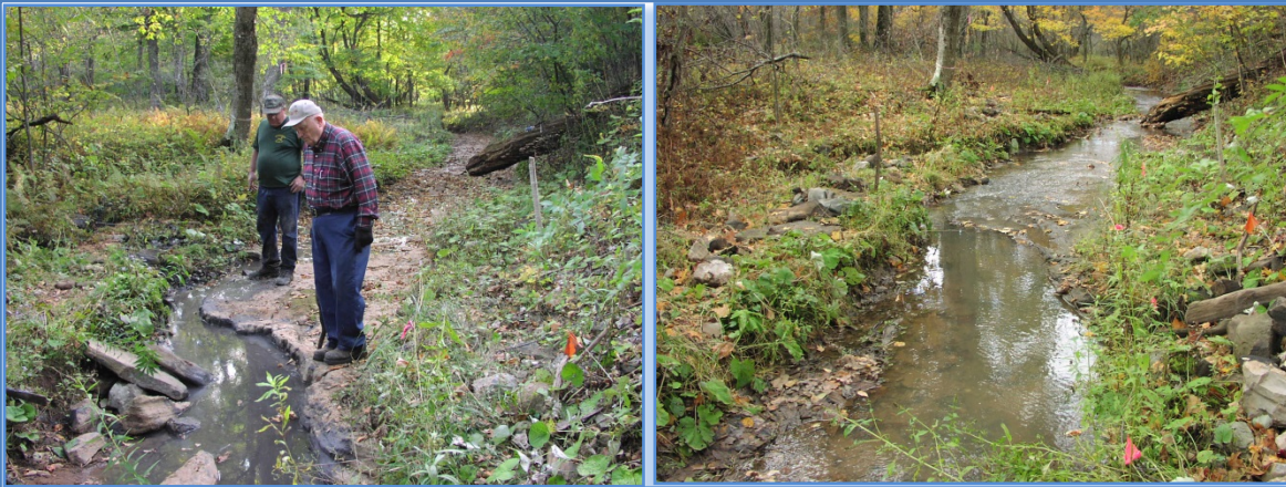
Photos During and Shortly After 2007 CCB-Grout Injection at Hoyes Run. Stream flow was restored within hours of grout injection.
