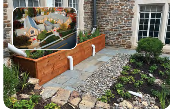
Parishioners take solace in the rain gardens installed at the Towson Presbyterian Church's courtyard; gardens feature native plants and will improve stormwater management and attract pollinators.
