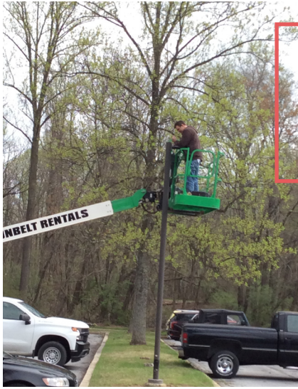
MPT master electrician Mark Duby performs some FY21 outdoor tune-up by installing energy-efficient LED light heads on the main parking lot. Over the past four years, the network's Facilities unit has upgraded all the Owings Mills campus parking lots' lighting to LED with further upgrades to come in FY22.
