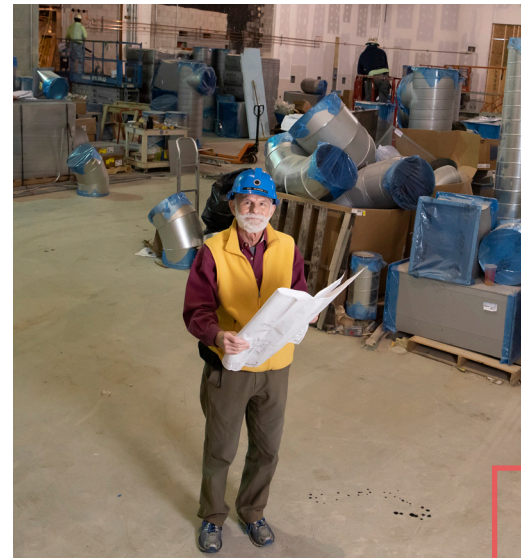
MPT's chief technology officer, George Beneman, on the Kaplan Studio construction site.
