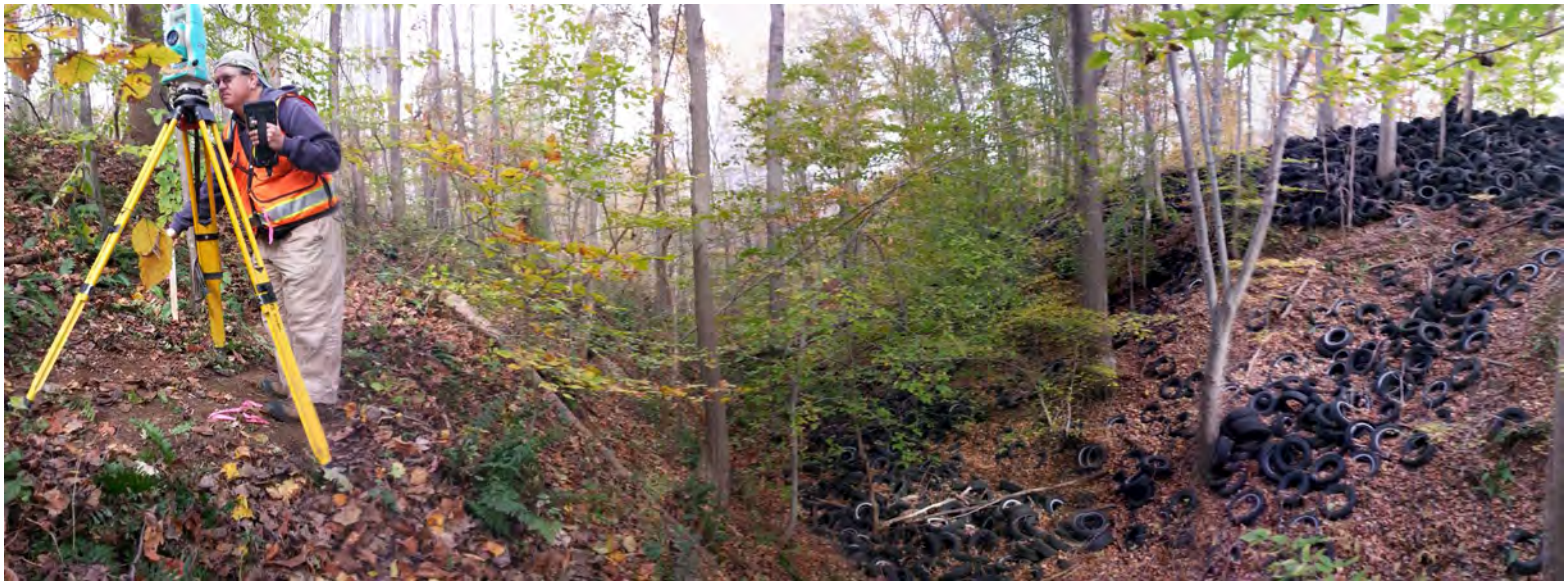
Wetland and forest services at the Boehm scrap tire clean-up site
