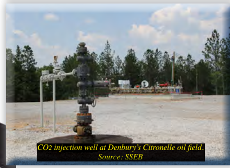
CO 2 pipeline extends from Plant Barry to the Citronelle oil field. Source: Denbury Resources Inc.
