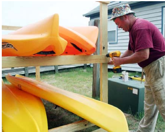
John Day Jr. works on a rack that was built to hold the rental kayaks at Breezy Point Park. The kayaks can be rented by the day or the hour.
