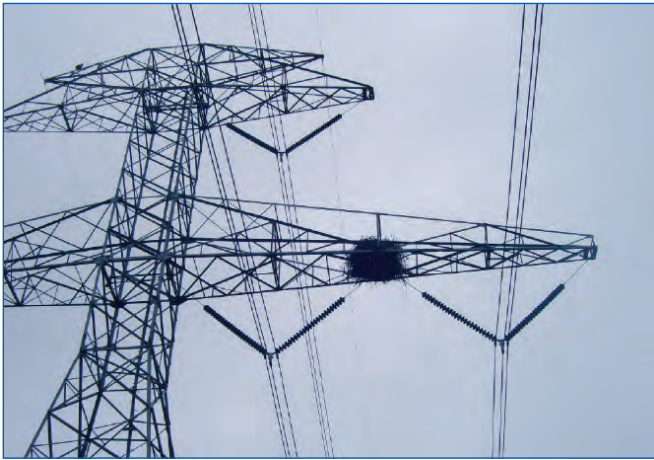
Figure 4-31 Eagle's Nest in a Transmission Tower
