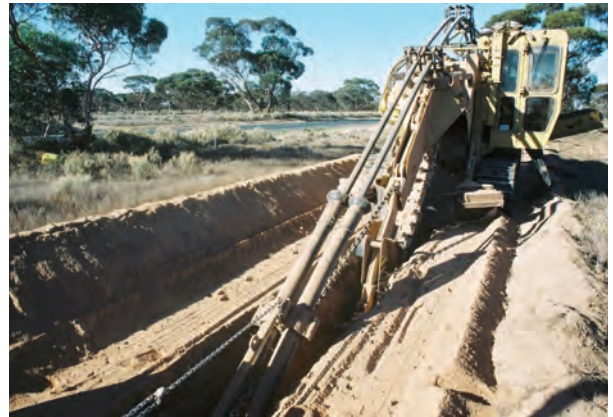
Figure 2-22 Direct-burial Underground Transmission Line Installation
