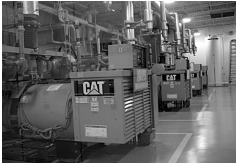
East Kentucky Power Cooperative's Bavarian Landfill Plant in Boone County, Kentucky. The Plant utilizes the methane gas from decaying municipal waste to produce electricity for more than 3500 households in northern Kentucky.
